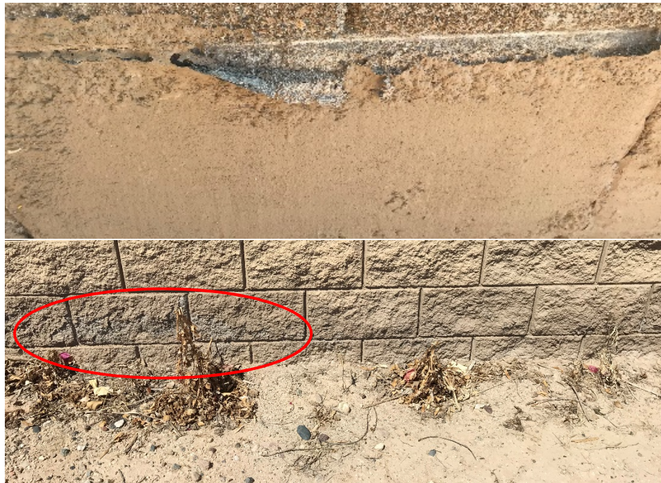
Figure 8. Examples of Loss of Paint and Surface Degradation
