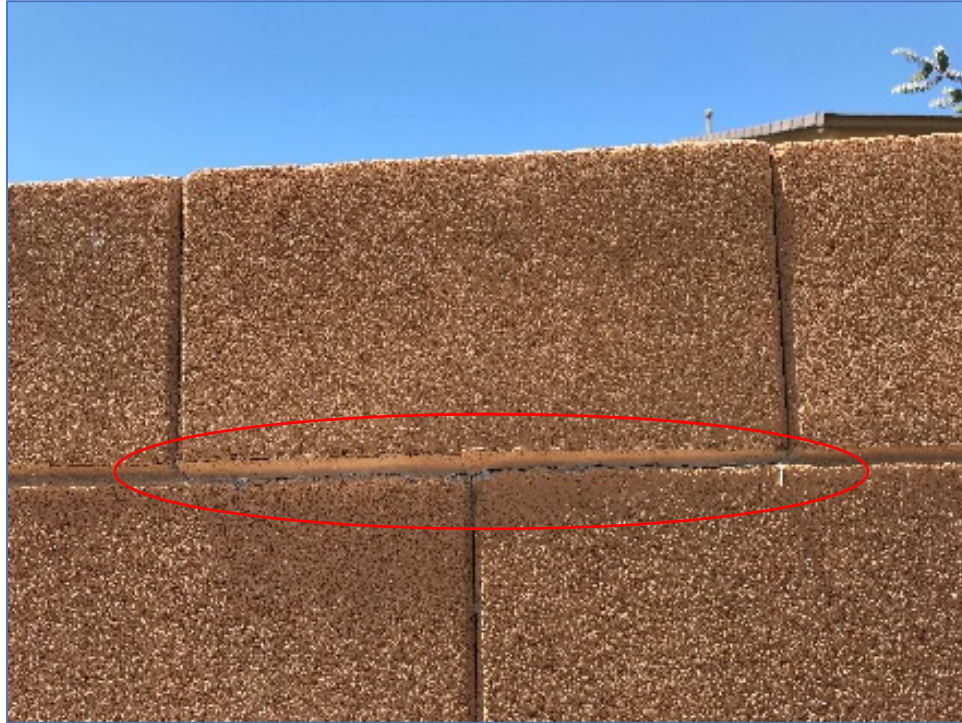
Figure 9. Example of Loose CMU
