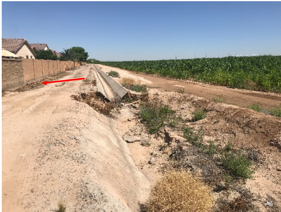
Figure 12. Ground sloping towards wall - Wall at South End
