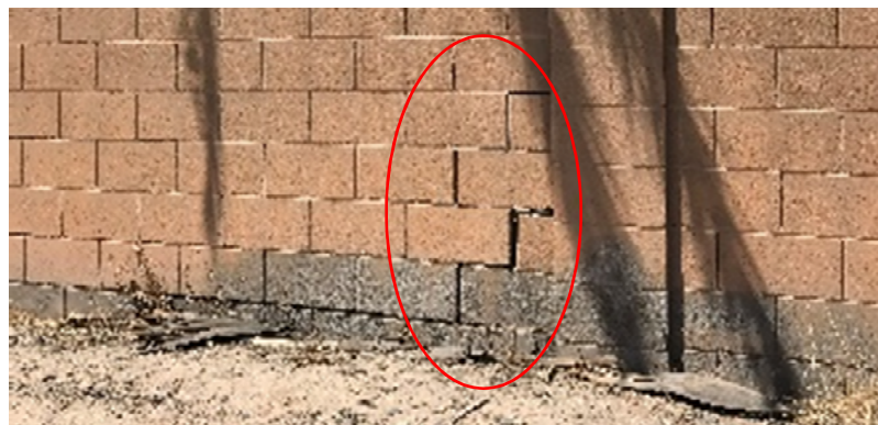
Figure 10. Examples of Cracking
